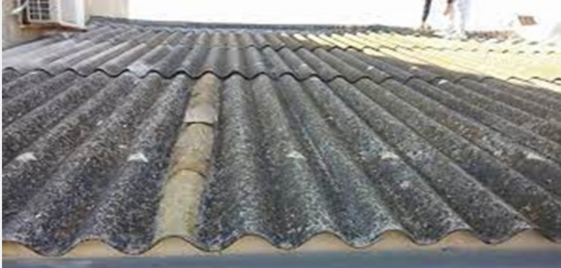
Figure 1: Asbestos sheet used as a roof or shed, with a corrugated shape imitating a tiled roof (Elenit).
